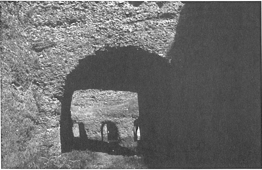
Fig. 14. The Negub tunnel, which supplied water from the Greater Zab to the Patti-hegalli canal, photograph from the west.
